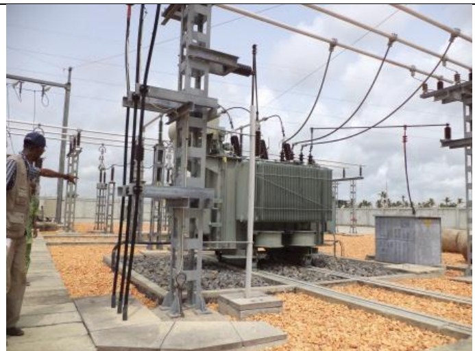
Poste de Transformation_Site_SBEE_SEME
